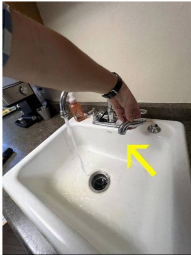
Kitchen sprayer not working
