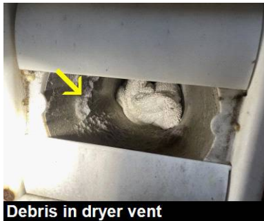
Debris in dryer vent
