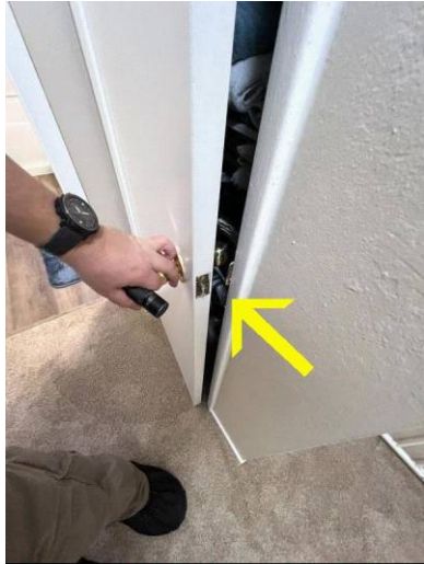
Upper hall closet door does not latch
