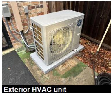
Exterior HVAC unit
