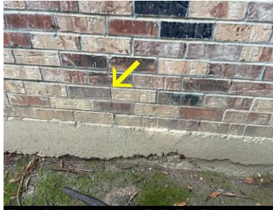
Crack in veneer @ left of home
