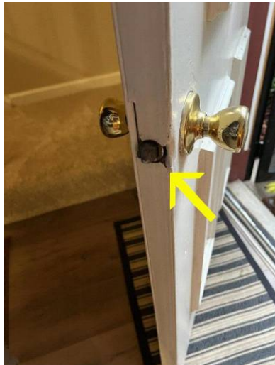
Damage @ entry door
