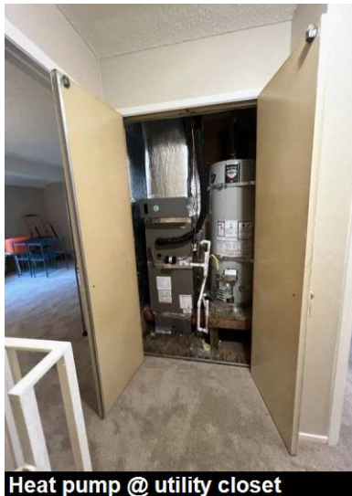
Heat pump @ utility closet Advanced Distributor Products.
