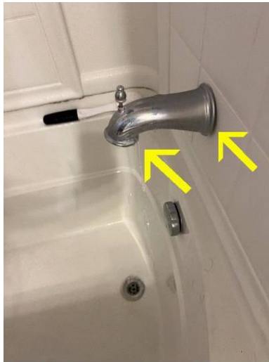
Leaking diverter & missing caulking
