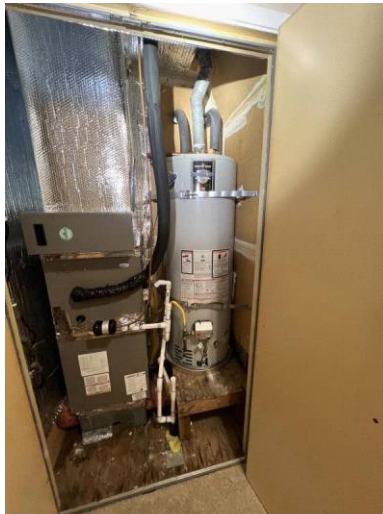
Water heater @ upper hall closet
