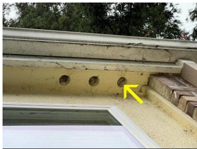
Paint & debris @ soffit vents
