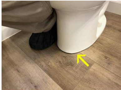
Loose toilets in home
