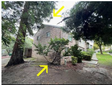
Tree & plant too close to home
