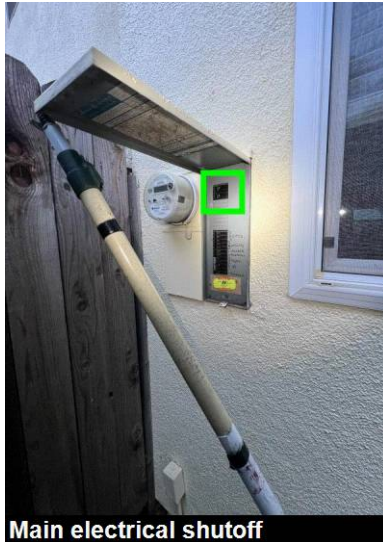
Main electrical shutoff
