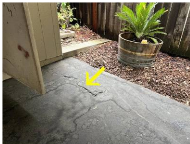
Cracks in asphalt
